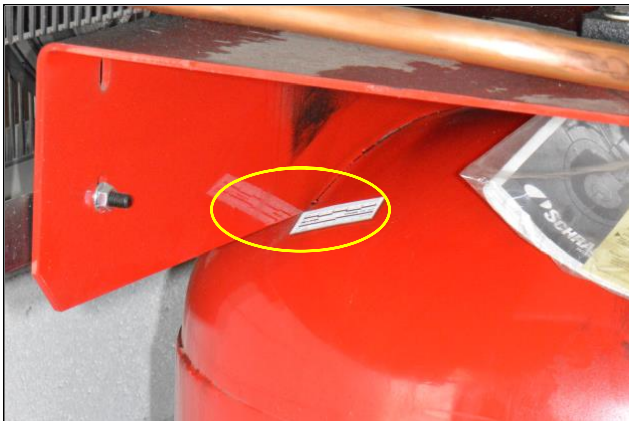
Figure 3. One of the four corners where the welds attach the compressor mounting bracket to the top head of the tank.
